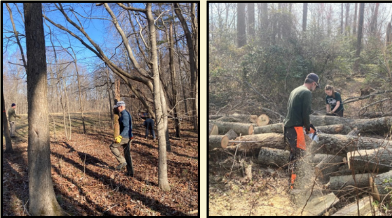
Left: Volunteers remove vegetation from the Greg & Tamea Bowen memorial area, which is under construction. Right: Dale Hutchins and Addie Brown cut downed trees on Horse Swamp Trail.
